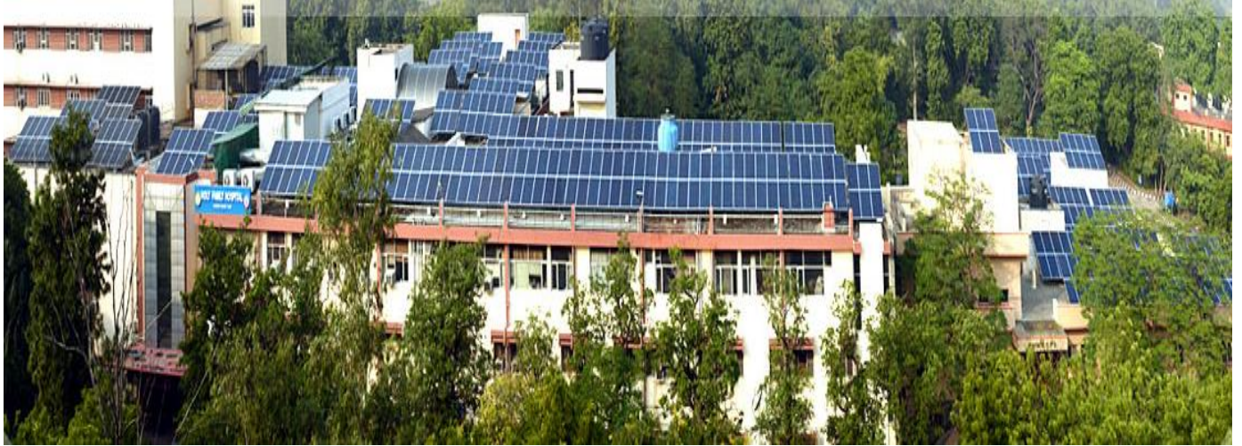
Fig 1: Rooftop solar panels at the Holy Family Hospital building 3
