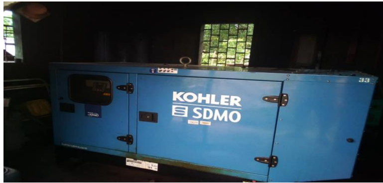
AN OLD GENERATOR AT NGOUNSO BAPTIST HEALTH CENTER
