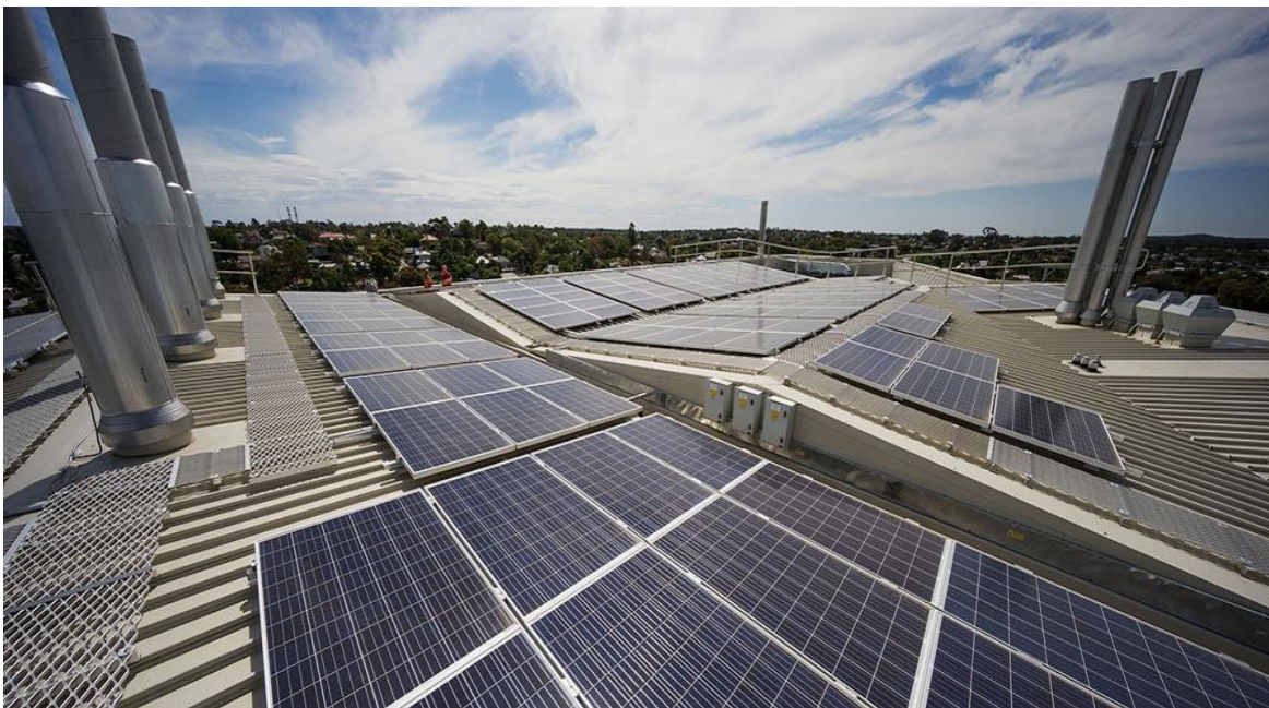
Image: Solar array on Bendigo Hospital roof
